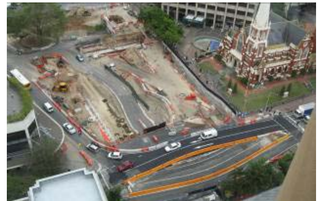
Top: Windsor Rd North West Connect Alliance, QLD Bottom: Inner Northern Busway, QLD
